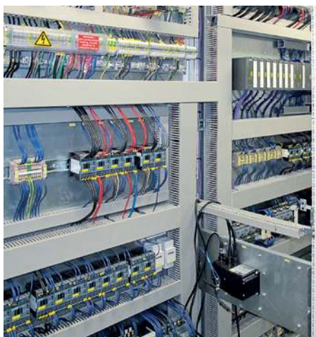
↑ High quality components in the electro-container
