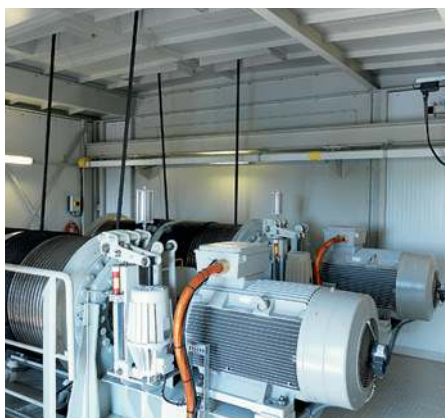
↑ Machinery room: spacious and maintenance-friendly
