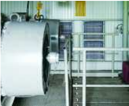
Spaciousness of the machinery house grants good accessibility and easy maintenance
