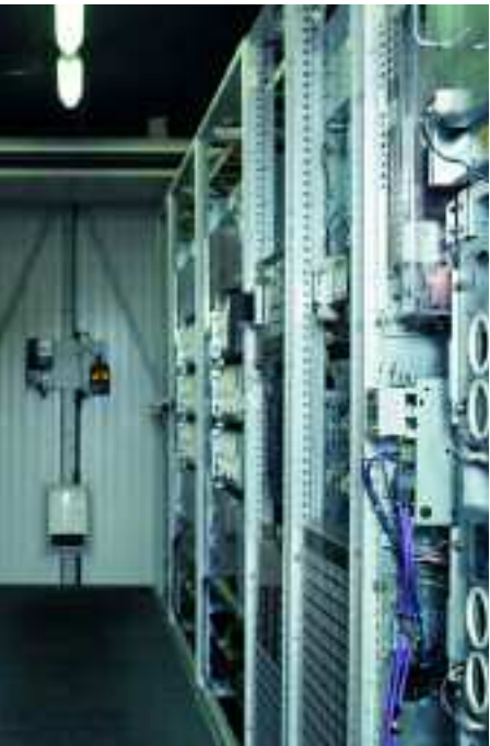
Open racks for electrical equipment are common
